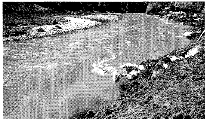
Chalk Creek-- one of several water quality improvement projects successfully completed by the Division of Marketing and Conservation. The streambanks were stabilized with specially placed rocks and deep rooted vegetation.
